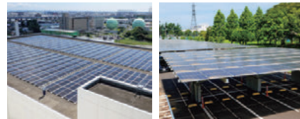
Solar panel at Shizuoka Plant Solar car ports at Ibaraki Plant
