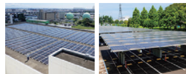
Solar panel at Shizuoka Plant Solar car ports at Ibaraki Plant
