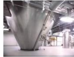
The depreciation period for SD facilities is around eight years, and the operating period is approximately 20 years
