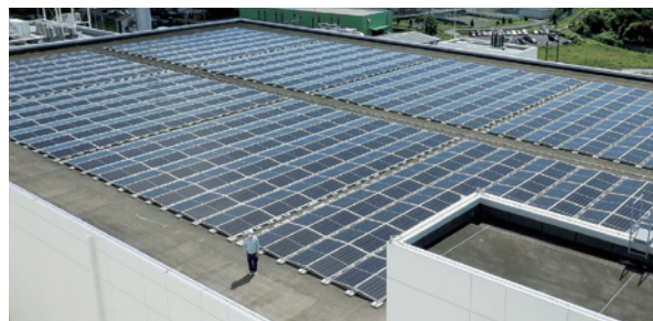
September 2021: Solar panels installed on the crude drug warehouse at the Shizuoka Plant
