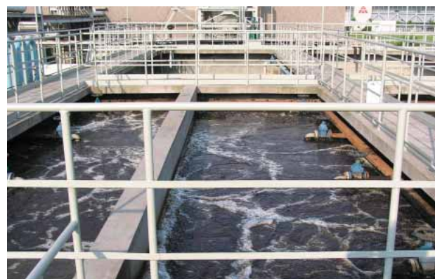
▲ Waste water treatment facility (Shanghai Tsumura)
