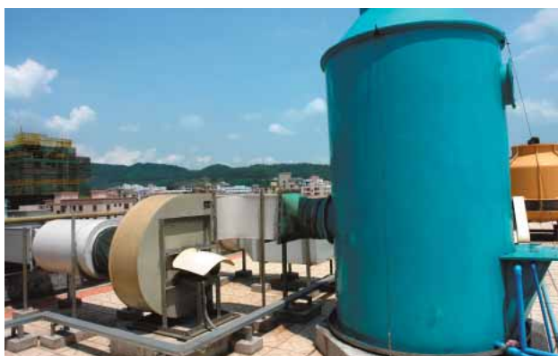
▲ The purification of the exhaust with water scrubber and the photocatalyst (Shenzhen Tsumura)
