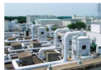
▲ Water Scrubber at the laboratory
