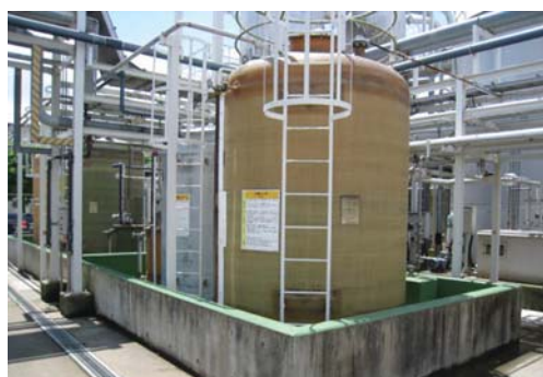
Dike for a caustic soda tank at the Ibaraki Plant
