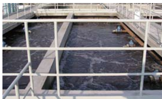
Effluent treatment facility (Shanghai Tsumura)
