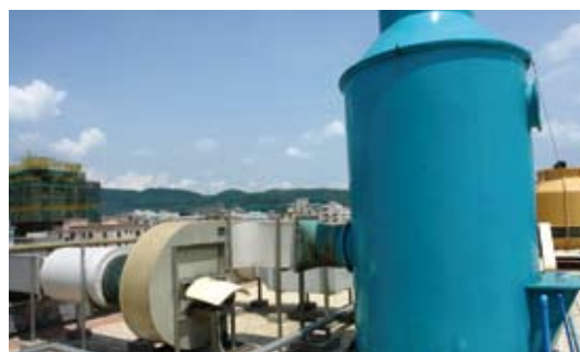
Water scrubber (Shenzhen Tsumura)
