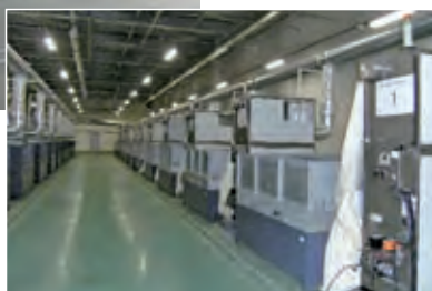
The processing plant for botanical raw materials
